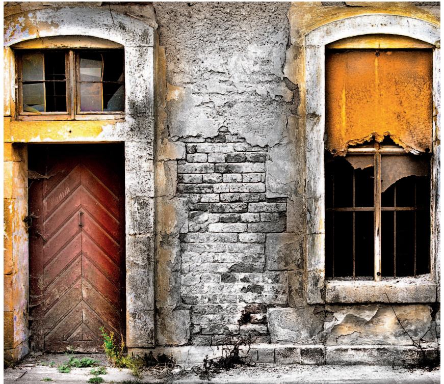
A commercial property in disrepair could cost the tenant dear
